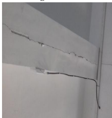
Damaged Expansion Joint
