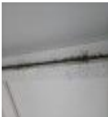
Damaged Expansion Joint
